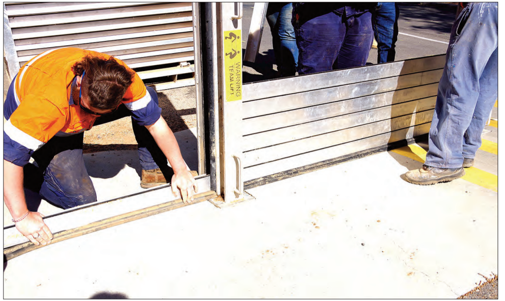
• Buloke Shire Council staff practiced deploying the mechanical flood barrier in Donald early on Thursday morning, ensuring staff are prepared to protect the community during flood events.
