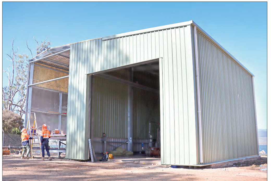
• Lake Fyans Pump Station.
